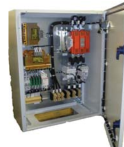
Pinfabb Q-05 Box Start Pumps
